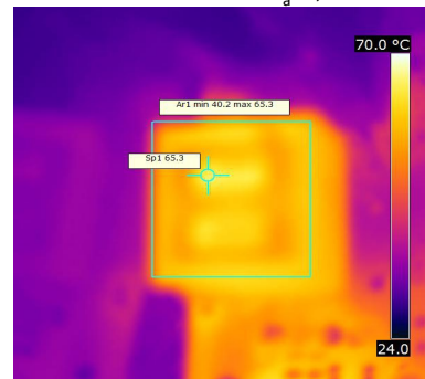
Itacoil transformer – t a 27,0°C
